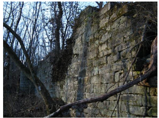
Remains of the Ashland Iron Works are still visible in the woods behind Ashland today.
